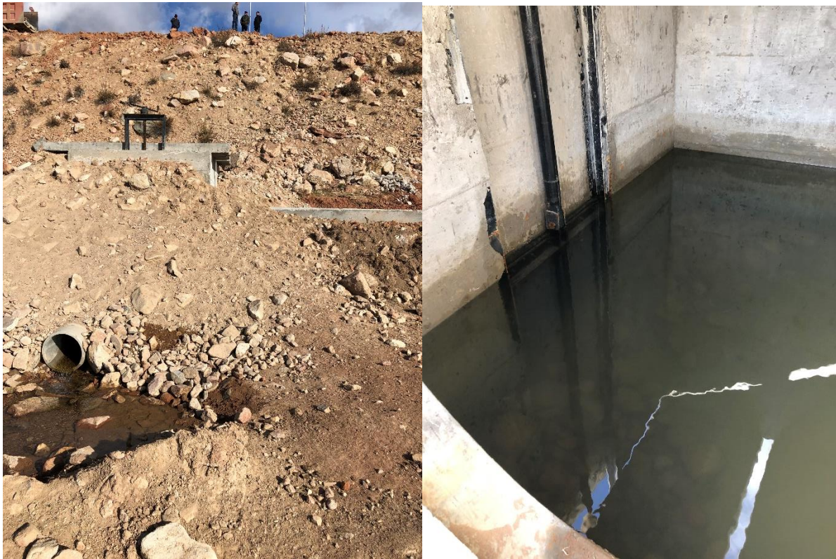
Water Seeping From the Outlet Works Through the Relief Gate (Left). Water in the Outlet Structure Overtopping the Closed Slide Gate (Right)
