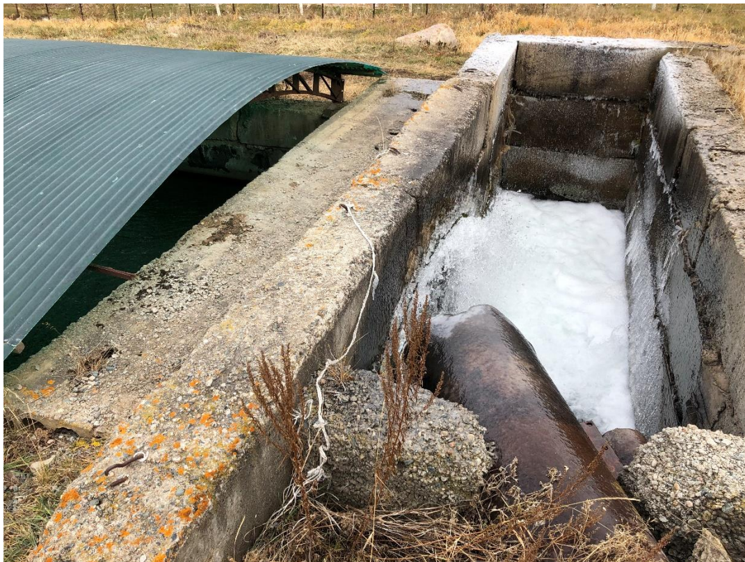
Gravel Filter Facility (Above and Next Page)
