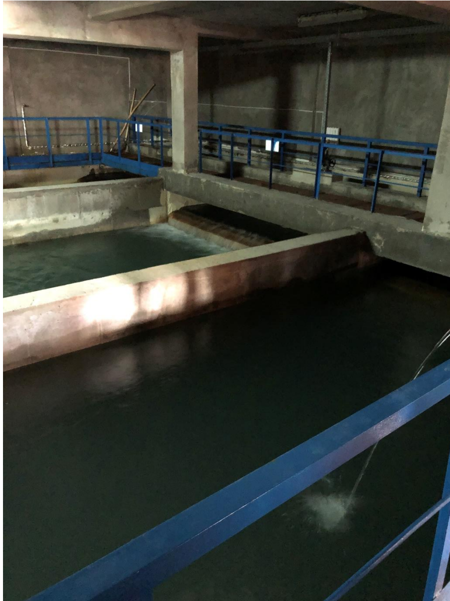
Interior of the Water Treatment Facility
