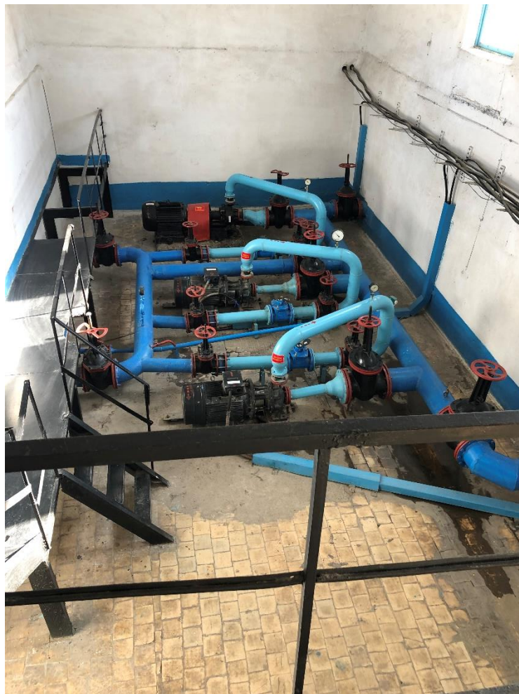
Third Lift Station
