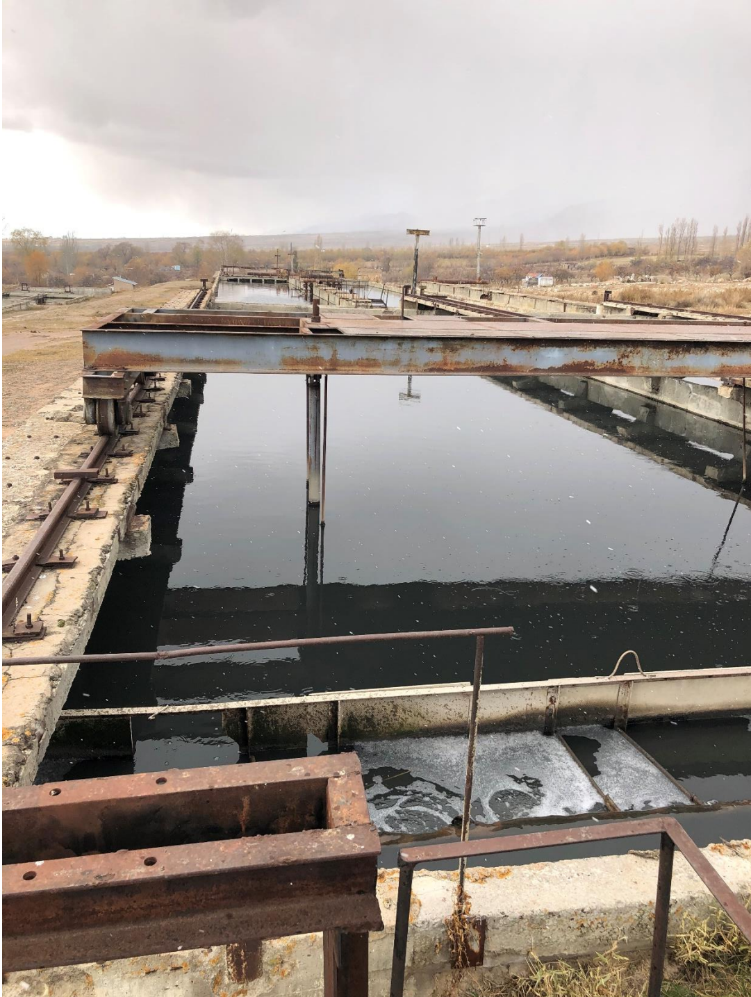
Wastewater Treatment Facility Near Cholpon-Ata
