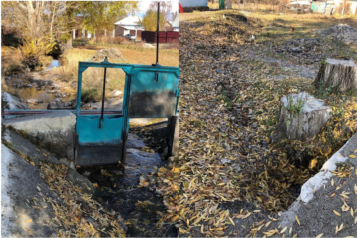
Ditches and Laterals in Karakol in a Poor State of Repair
