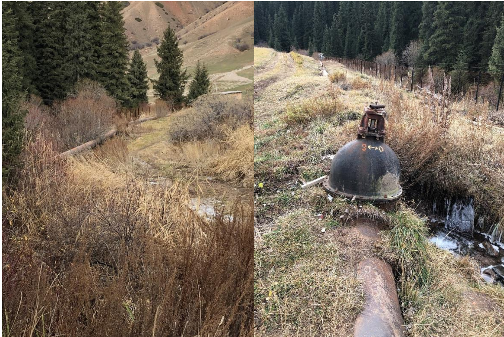
Pipe and Relief Valve Leading to Gravel Filter Facility
