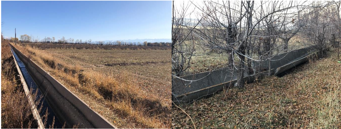
An intact above-ground concrete irrigation ditch (left) and a more typical derelict one (right)
